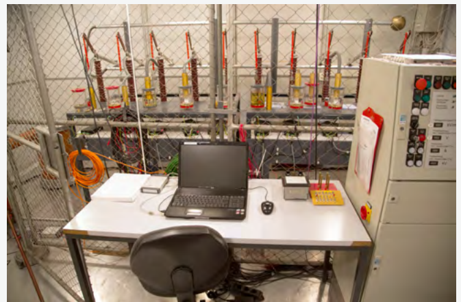
PARTIAL DISCHARGE MEASURING CABIN
