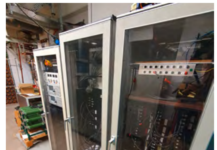
LVDC CONTROL CABINETS WITH PASSIVE LOADS & CONTROLLED VOLTAGE SOURCES
