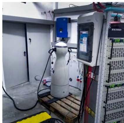
Figure 1: PION AG charging station in the 7-hour 44kW continuous load test
