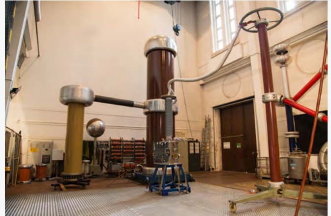
AC VOLTAGE TRANSFORMER
