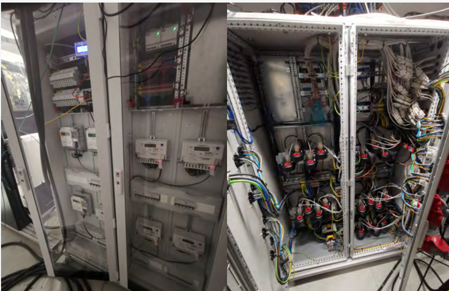
Meter measurement cabinet for the development of measurement methods for multiple use of PV home storage systems with an output of up to 70kW; Project MELANI
