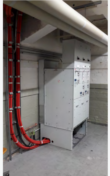
SUBSTATION FOR CONNECTION TO THE 6 KV UNIVERSITY NETWORK OR 20 KV NETWORK OF THE MUNICIPAL GRID OPERATOR.
