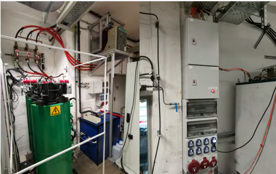
6KV supply with two safety circuits and control of a top switch, a safety disconnect, an earthing disconnect and a load-break switch; Project SMS2
