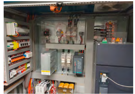
LVDC CONTROL CABINET WITH LVDC-AFE & DC BUSBAR
