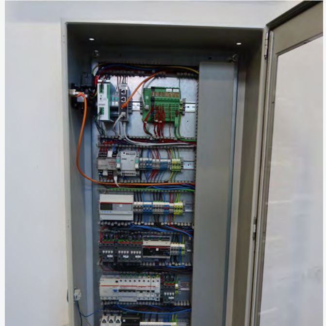
LABORATORY CHARGING STATION OF THE EMOBILITY PRACTICAL COURSE
