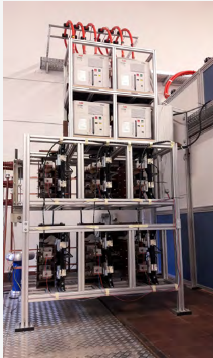
B12 RECTIFIER INCLUDING UPSTREAM CIRCUIT BREAKER
