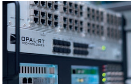
Figure 4: Powerful OPAL real-time simulator with analog interfaces for controlling components in the laboratory
