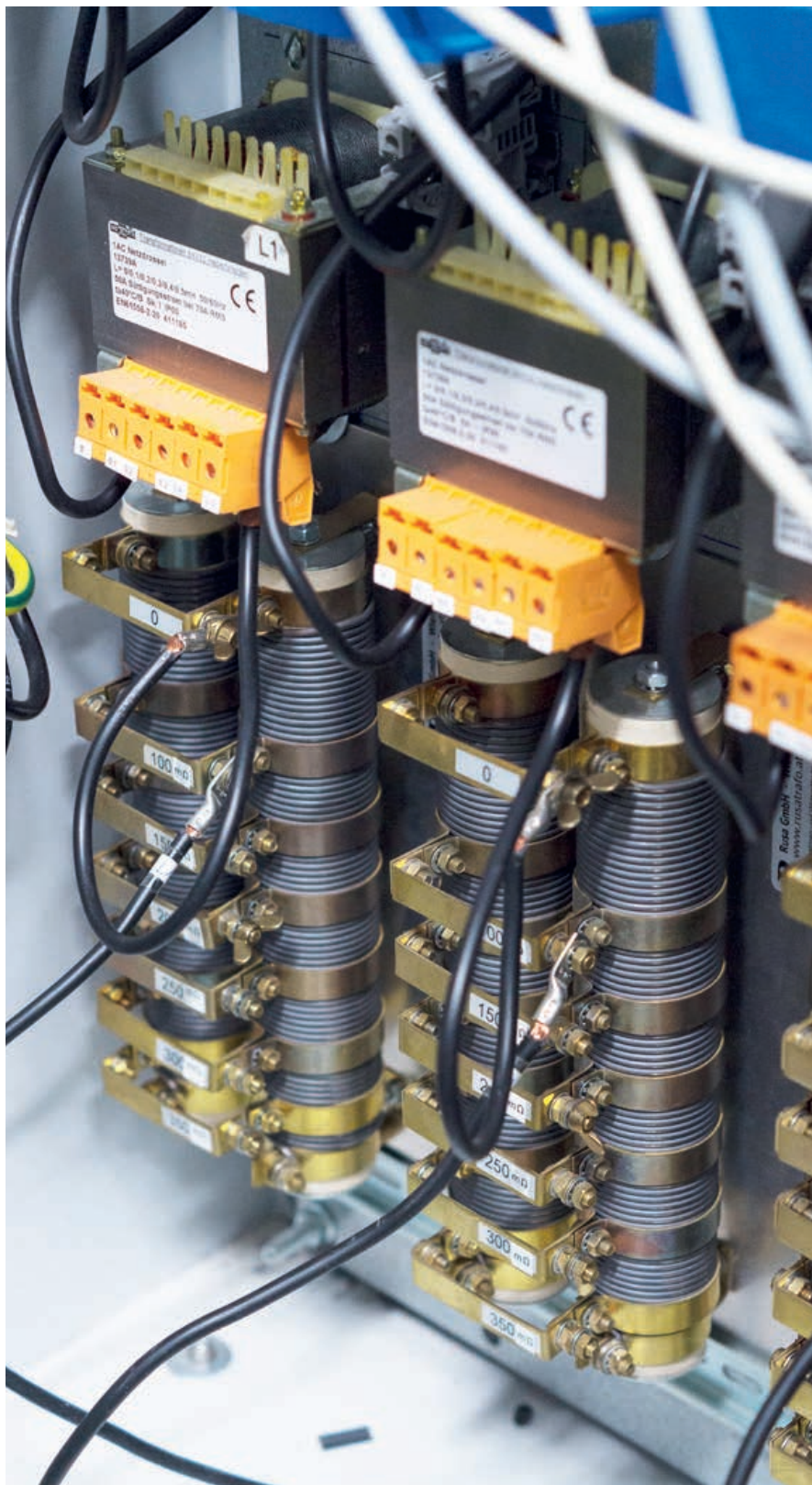
Figure 6: Line replicating elements correspond to up to 1.8 km of low voltage cable
