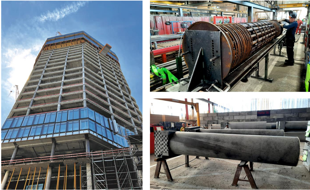
Figure 9-1: FOUR high-rise project in Frankfurt: precast columns installed in high-rise structure (left); reinforcement cage and finished column at SACAC AG in Lenzburg, Switzerland (right) [Emp-21]
