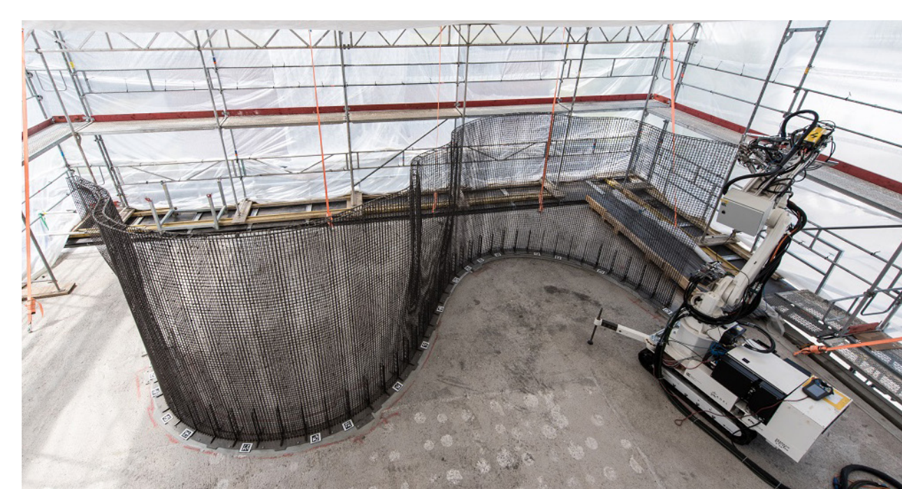
Mesh Mould, Phase 2: In situ fabrication of a steel mesh that acts as reinforcement and formwork.
